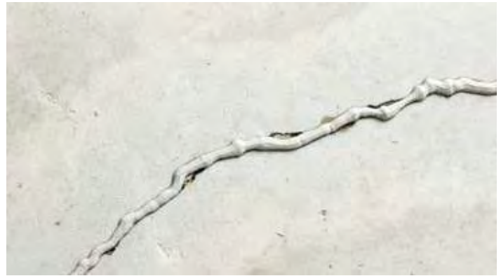
Crack filled with crack sealer
