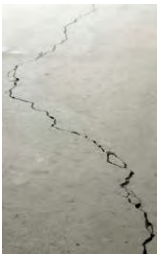
Typical concrete crack.
